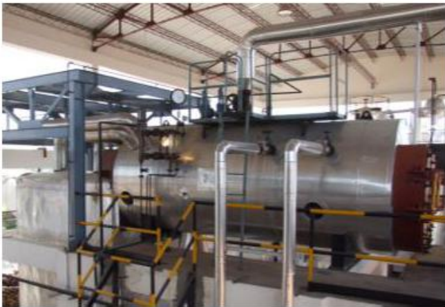
Agro Waste Fired Compo Boiler
